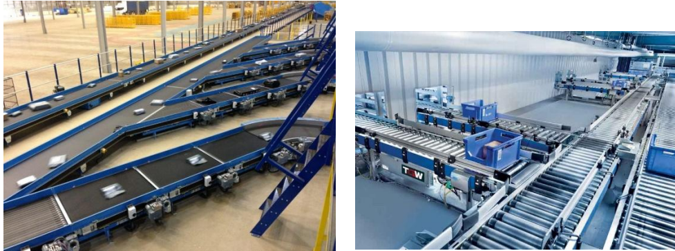
a) Belt conveyors, source: [12]
